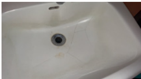
Krakelering i servant.
