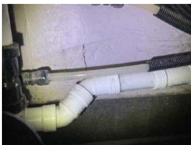
Sprekk i malt plate under servant.
