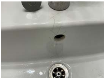
Krakeleringer i servant.
