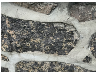
Sprekker i murfuger
