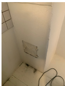
Manglende ubrennbar plate under sotluke
