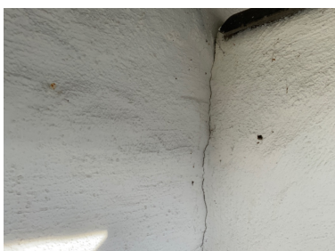
Sprekker i overgang vegg/mur
