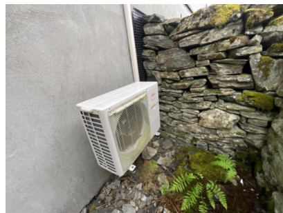
Varmepumpeaggregat (Fujitsu), langsida mot vest
