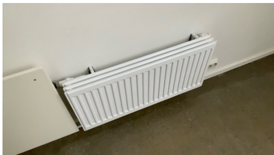
Radiator i stue.
