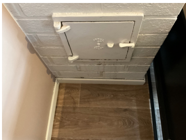
Manglende ildfast plate under sotluke.
