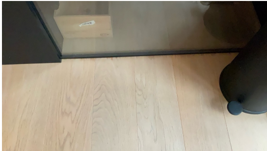
Fuktskade i parkett under glass.
