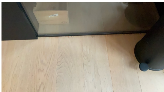
Fuktskade i parkett under glass.
