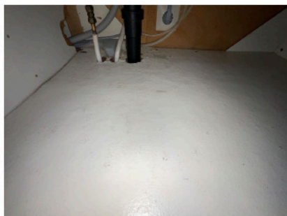
Fuktsvelling i plate under vask.
