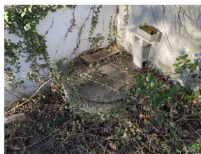
Eldre septiktank i betong.
